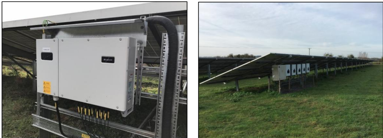
Plate 3.3 Typical String Inverter
